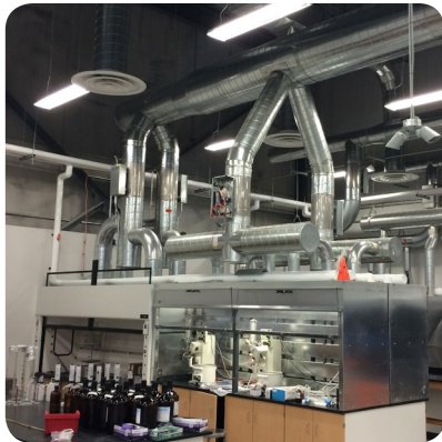
Top: MDCL 2nd Floor Fit-Out (McMaster University) Center: University Health Network Cyclotron Bottom: ALS Life Sciences Lab
